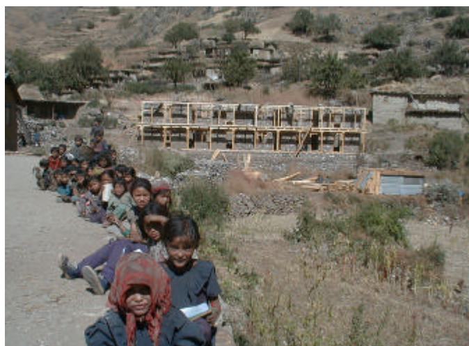
Plate 9: Chauganphaya hostel, mid-construction, 2001. These are the school children who will board in the hostel once completed.
