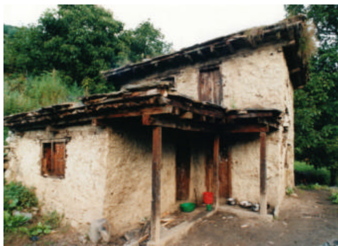
Plate 8: The current sub-health post at Syanda; this will be demolished to make way for the new sub-health post in 2002.
